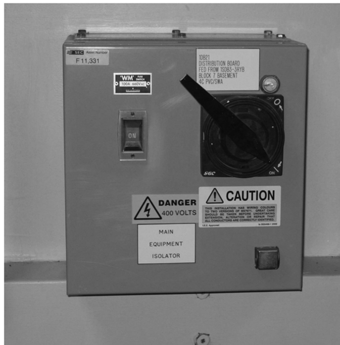
Figure 5.2 Mains supply switch.
